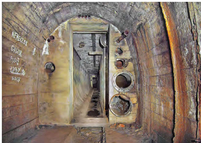
The way into the second bunker in the Schiller complex, with pipes for various services clearly visible
